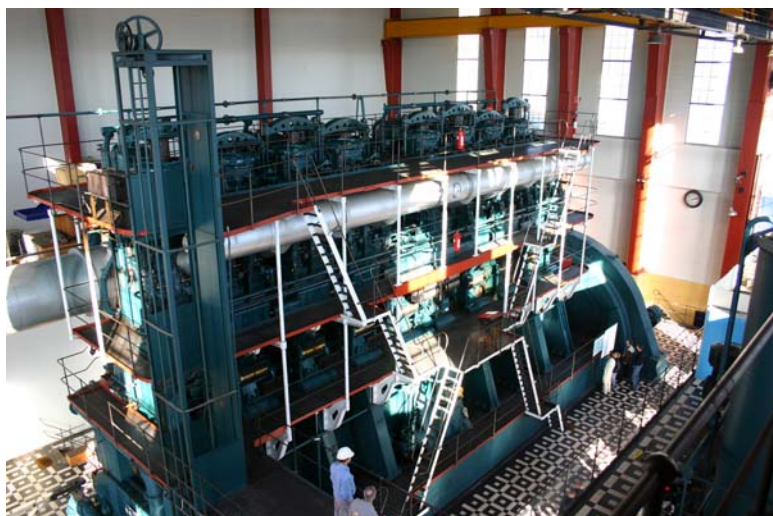
The 1932 B&W diesel engine at H. C. Ørsted Værket, which was the world's largest engine for approximately 35 years. It will be one of the main attractions in the new diesel science centre
